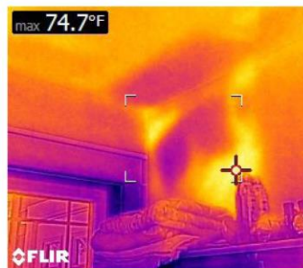
Missing Insulation – Summer Day E6 with MSX
